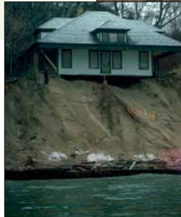
High lake levels on Lake Michigan in 1986 caused severe erosion.
